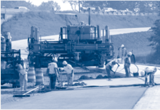
Construction crews begin paving the new exit ramp leading to State Route 58.
