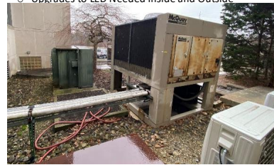
Admin Condensing Unit in Poor Condition and At End of Service Life
