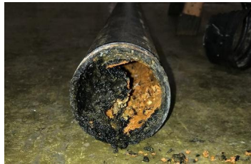
Deteriorated Cast Iron Piping from Admin Building During Recent Leak
