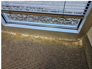
Water Infiltration at Window on Admin Building North Face
